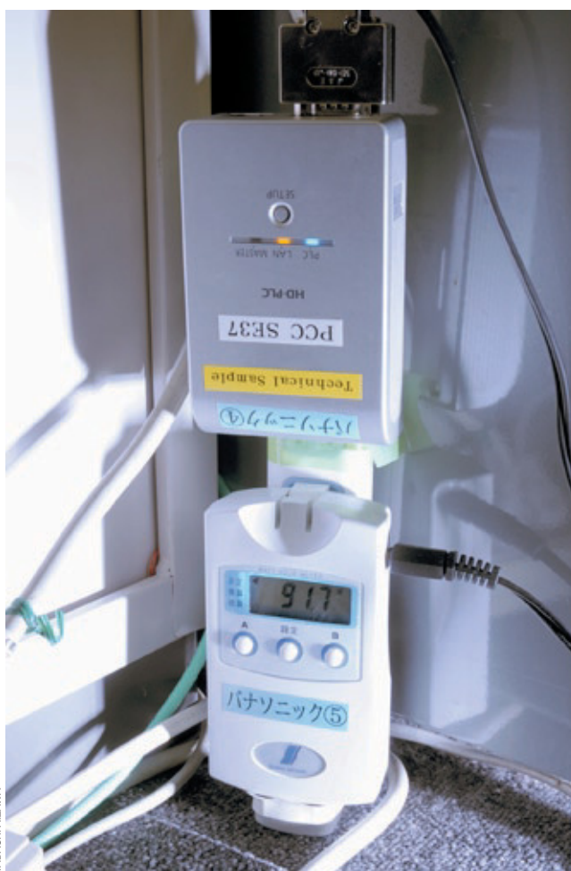
A measuring device to collect the data on electricity consumption of electric devices on a real-time basis
